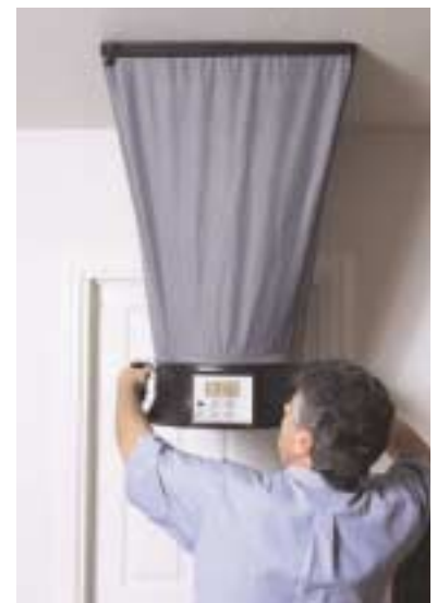
An airflow hood measures flow at the return vents.
